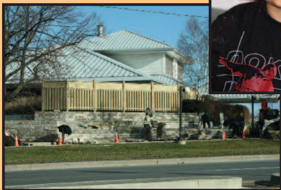
Necessary repairs were made to the retaining wall at West Division in Pickering.
